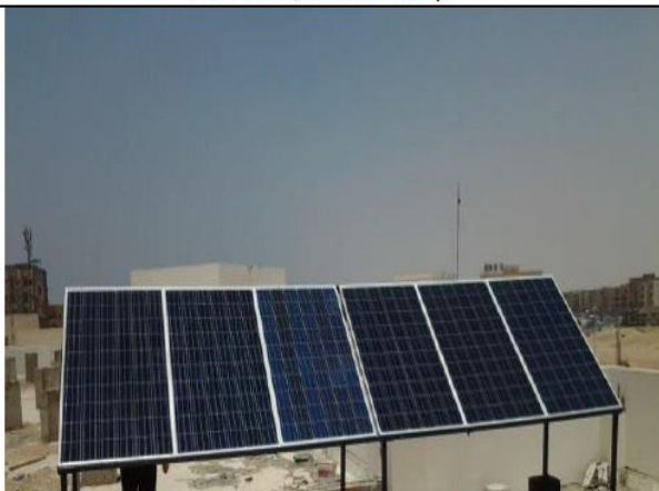
Example of 5 Kw Roof Panel (Beni-Suef University - Faculty of Postgraduate Studies for Advanced Sciences, Beni-Suef)
